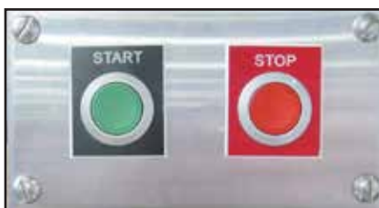
Fig. 15 - Pulper System Start/Stop Station
