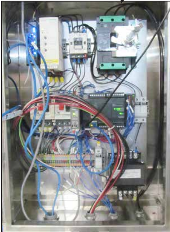
Fig. 7 - Main control cabinet power connection.
