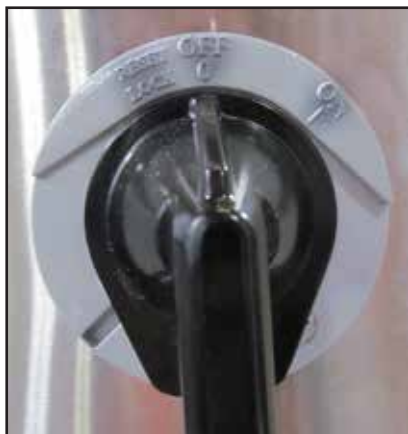
Fig. 13 - Circuit Breaker has On, Off, & Reset/Lock
