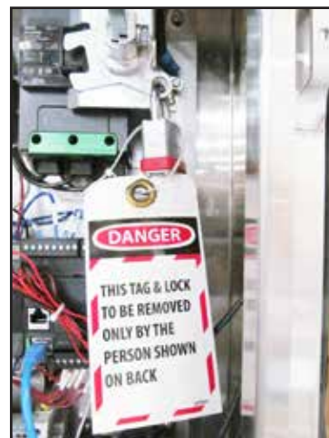
Fig. 14 - The circuit breaker should be locked and tagged when the panel is serviced.
